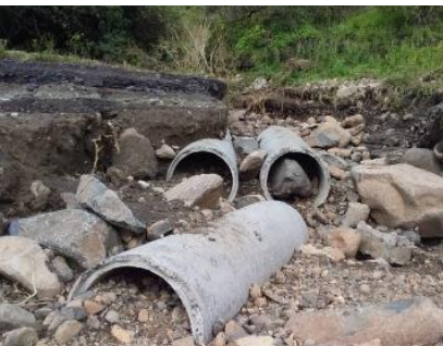
Mashunka Road washaway
